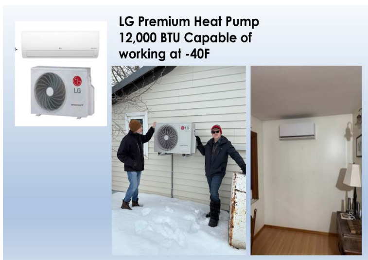
Figure 13. Heat pump demonstration in Kotzebue
