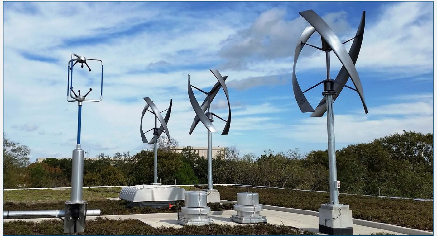
Wind Turbines at Building 12 NASA Johnson Space Center. Courtesy of Mike vanBavel / Dynamax Inc.
