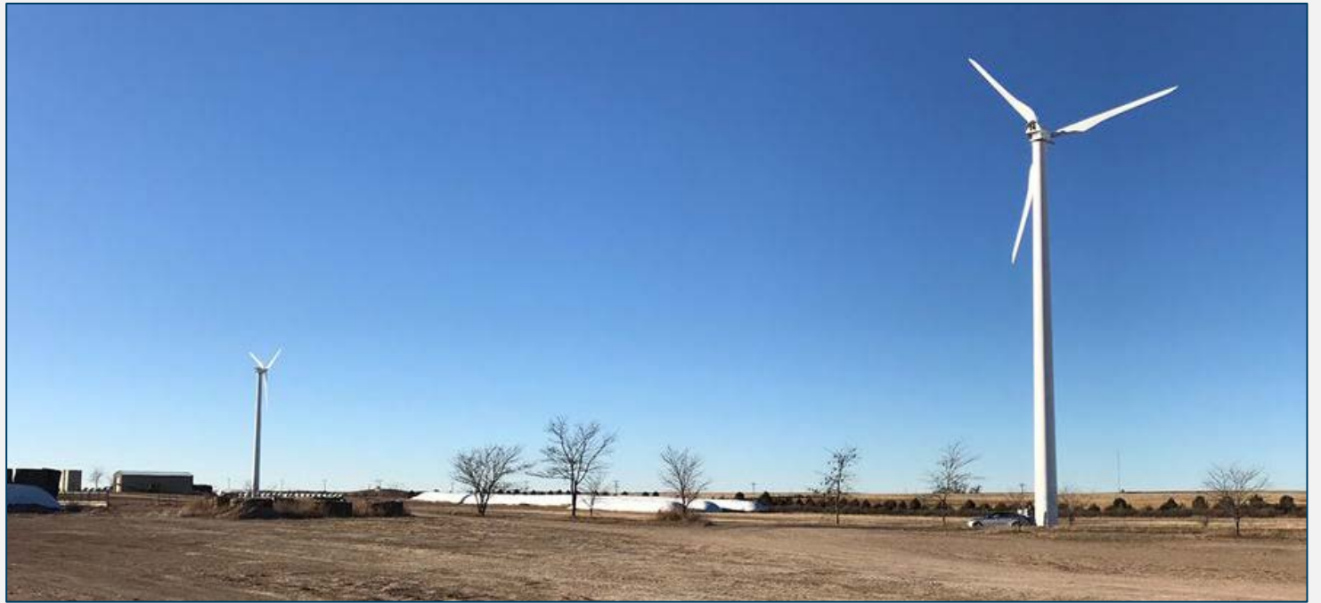
Two, 100-kW turbines in Yuma, CO. Courtesy Northern Power Systems
