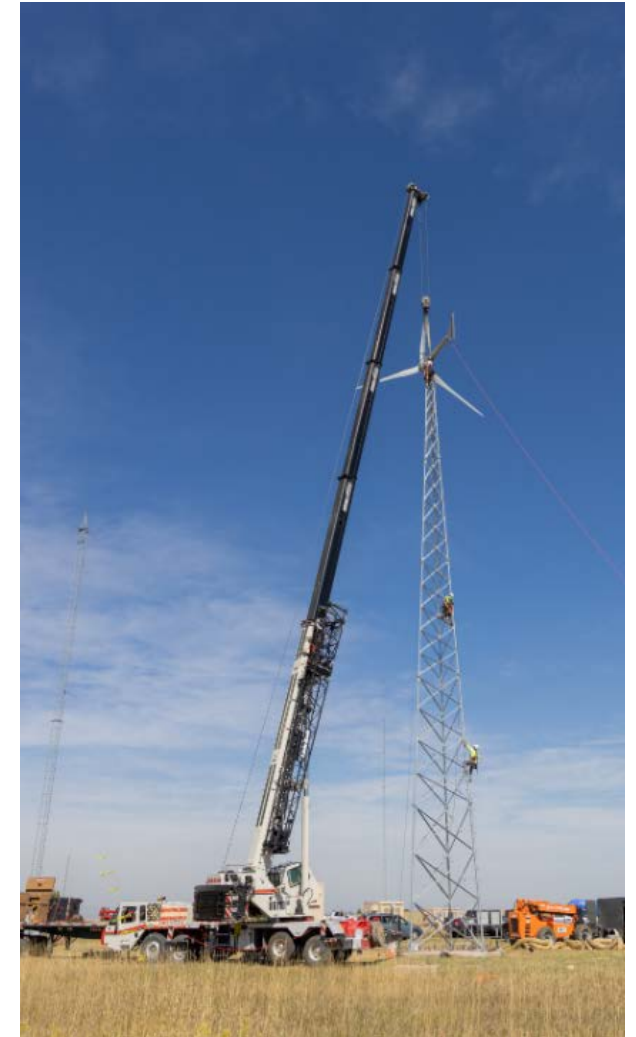
Bergey Excel 15 being installed at NREL's Flatirons Campus. Photo by Joe DelNero, NREL
