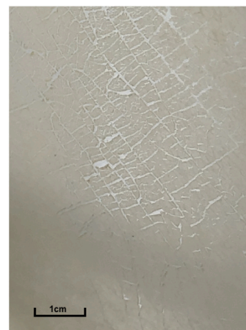
Fig. 5. Micro-cracks were observed from the site with ten years exposure. Site is located in Maryland within Cfa climate zone. The airside layer material is identified as PEN.
