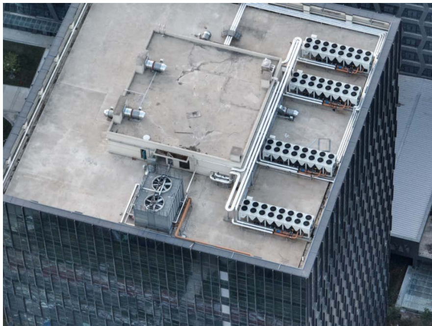
Figure 19. Example of buildings in the Electric Resistance Multizone Systems segment
