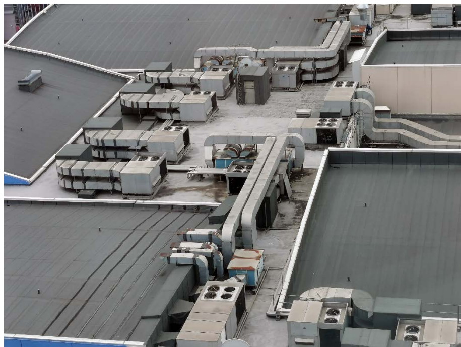
Figure 17. Example of buildings in the Packaged Multizone Systems segment
