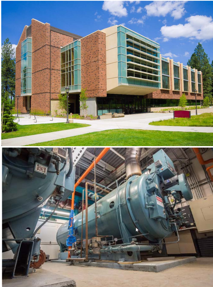
Figure 18. Example of buildings in the Hydronically Heated Multizone Systems segment
