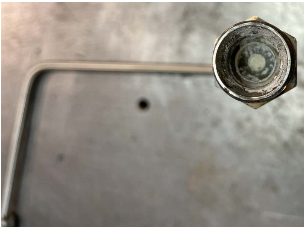
Figure 3.5.4-2. Salt condensation clogging exhaust gas line.
