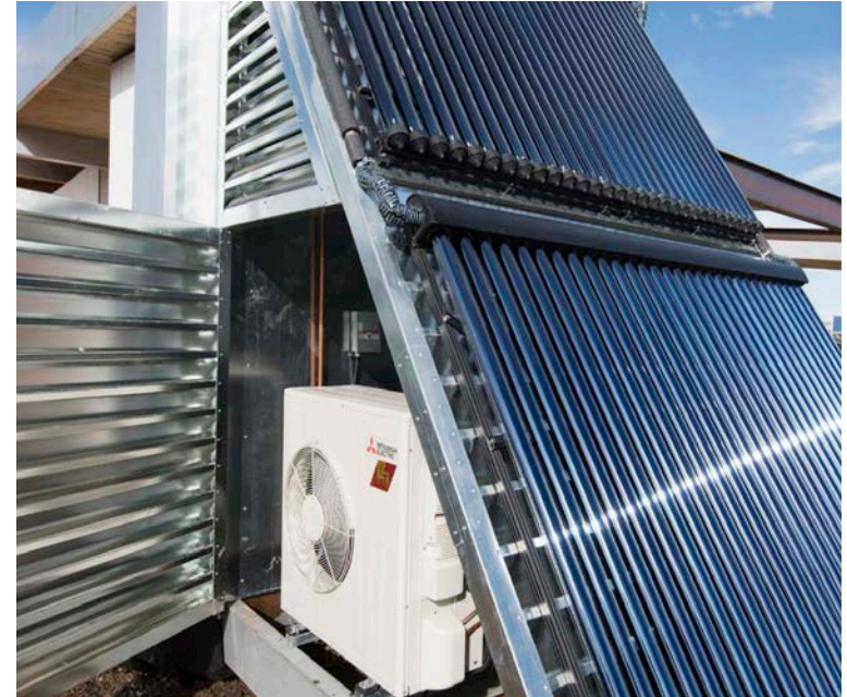
Non-concentrating solar hot water collector system. Photo by Dennis Schroeder, NREL 48515
