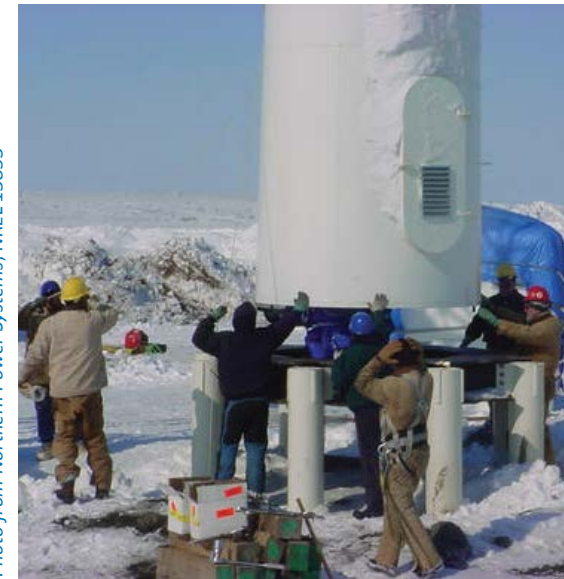
Photo from Northern Power Systems, NREL 13853
