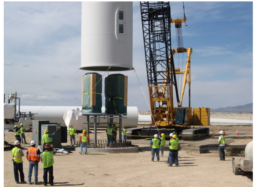
Photo from First Wind, NREL 16738
